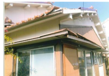
庇の腐朽・破損
