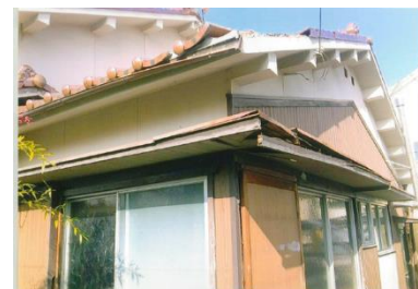
庇の腐朽・破損
